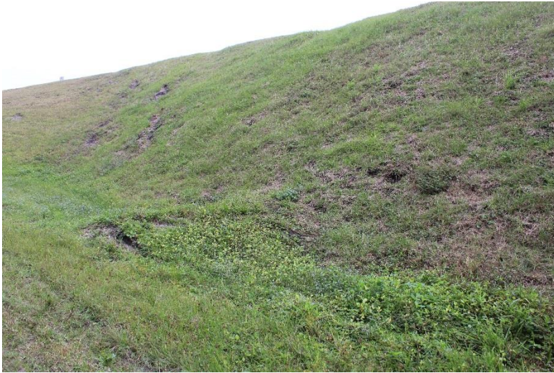
South Bottom Ash Pond (west side, looking northeast) Irregular rutting noted
