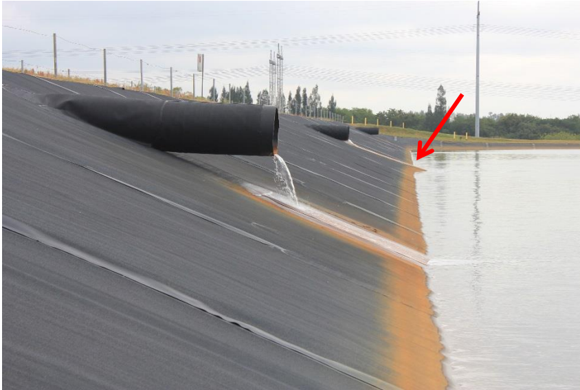
Long Term Fly Ash Pond (north side, looking east at bulge below central pipe from South Economizer Pond)
